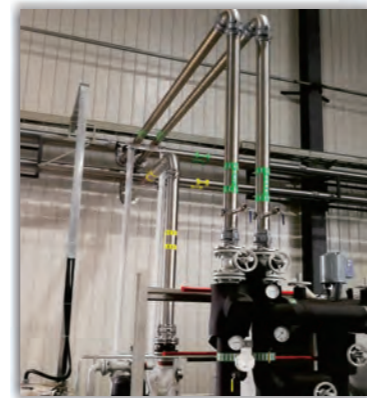
● Oil and Cooling water for Machinery.
