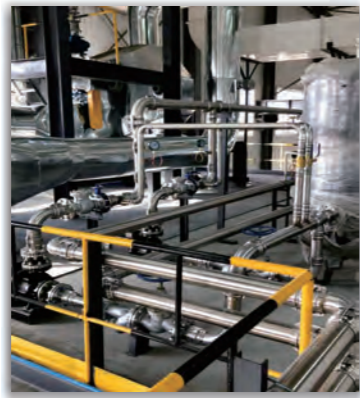
● Cooling water for new Material.
