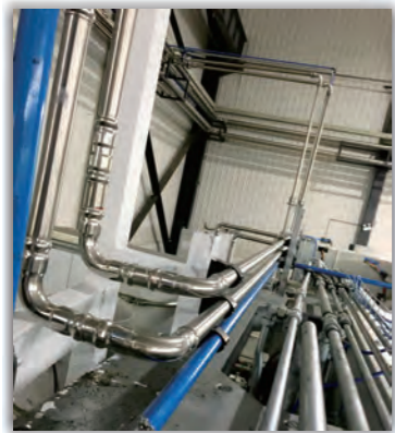
● Cooling water for Auto Parts.
