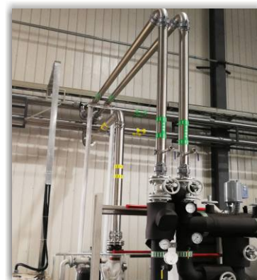
● Oil and Cooling water for Machinery.
