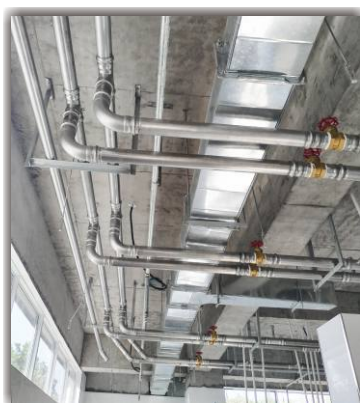
● Cooling water for IT industry.
