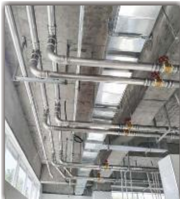
● Cooling water for IT industry.
