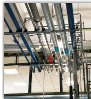
● Compressed Air, Nitrogen, Natural Gas, Oxygen, Argon, Cooling Water for LED.
